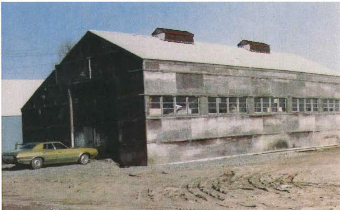
Building #33 before current metal cladding was added, 1984, Existing Building Inspection, Barry Wong
