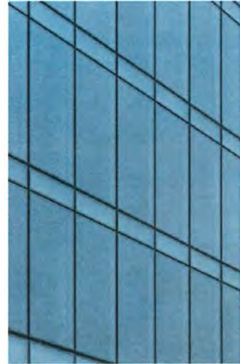
CW Curtain Wall Glazing w/ Mullion Caps
