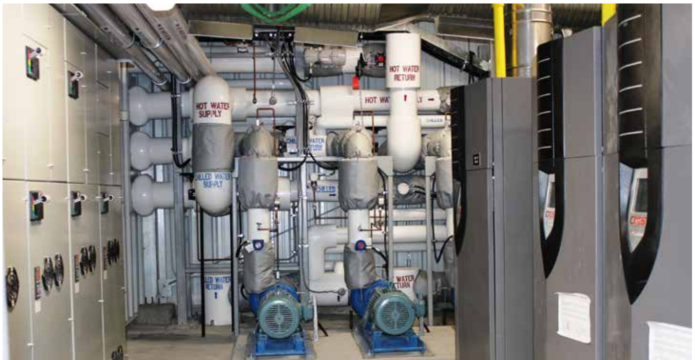
Alexandra District Energy Utility (ADEU) Phase 4 Expansion
