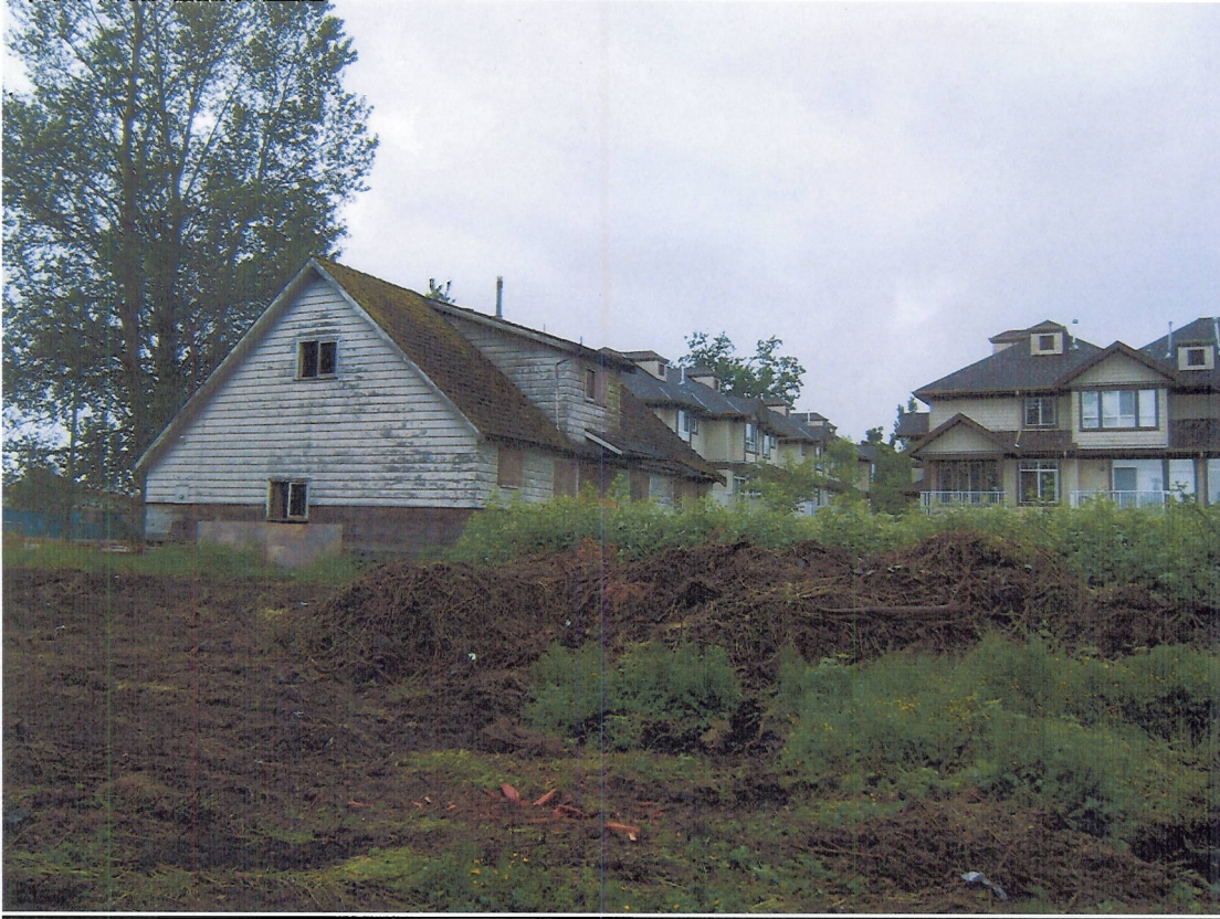
Address: 9611 ALBERTA ROAD- East side view of property) Taken by Ron Graham June 10 th , 2010.
