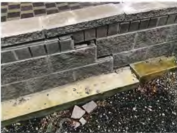
January 24, 2020 – failing decorative wall on property line adjacent to infill
