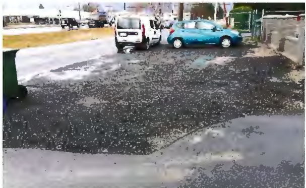
January 24, 2020 – Unauthorized Watercourse Crossing
