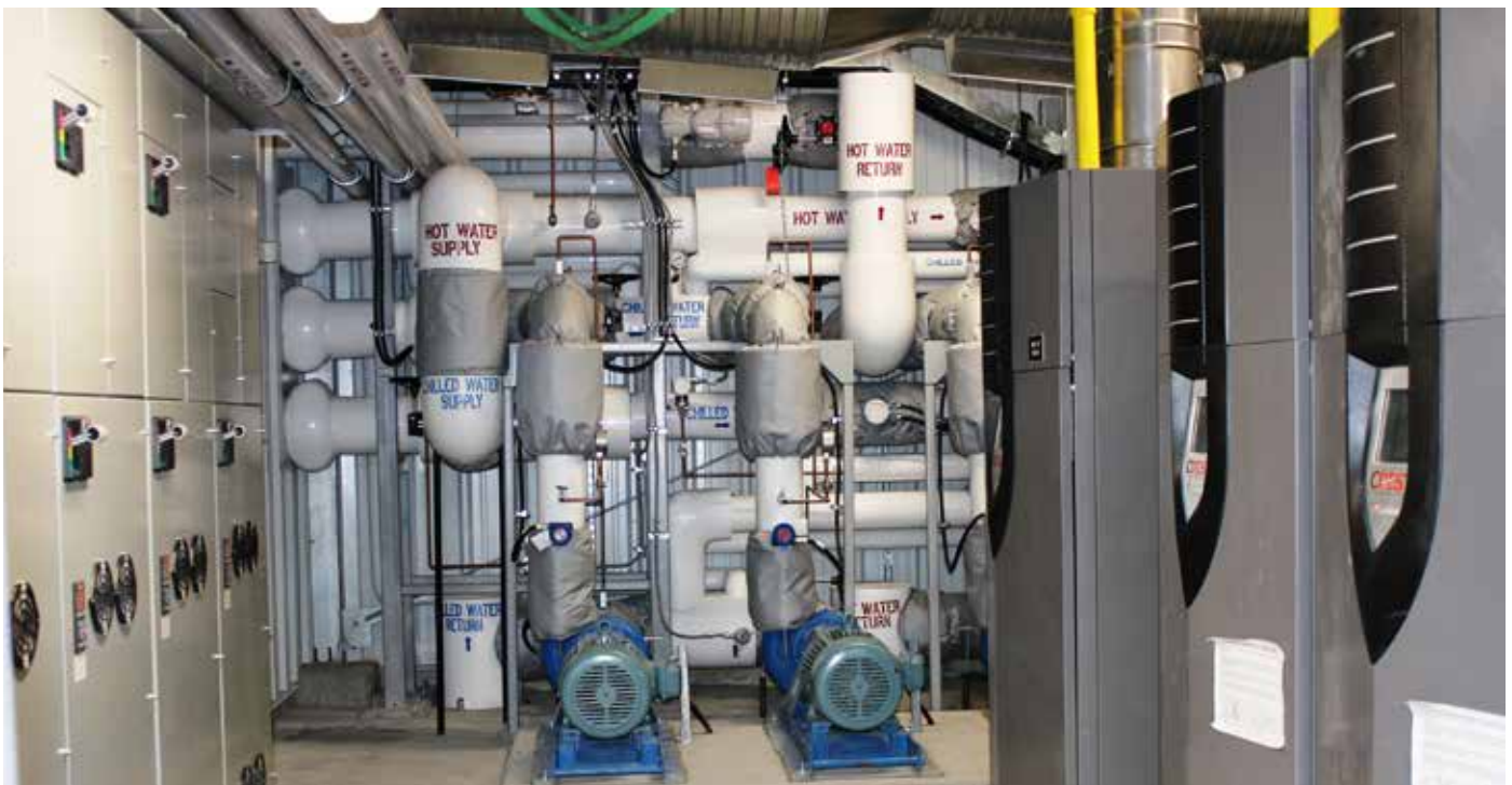
Alexandra District Energy Utility (ADEU) Phase 4 Expansion
