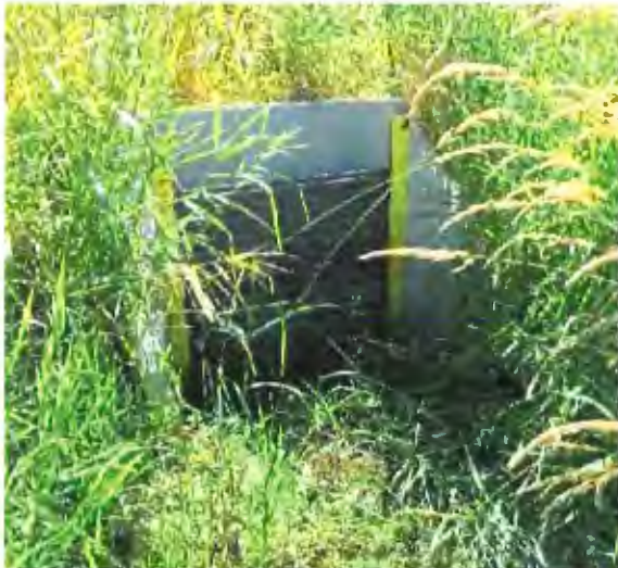
Figure 3-6: Stop log structure from front during dry season as modelled in Phases 2-4
