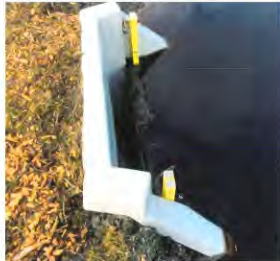
Figure 3-7: Stop log structure creating a weir outlet condition at the southern end of the bog site
