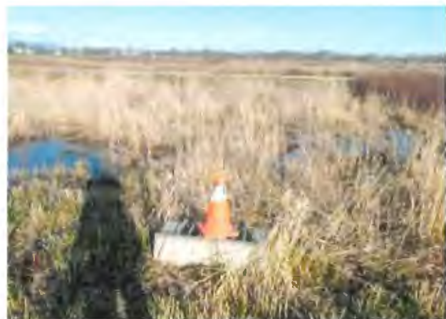
Figure 3-3: Present day headwall control structure installed north of Lansdowne Rd.
