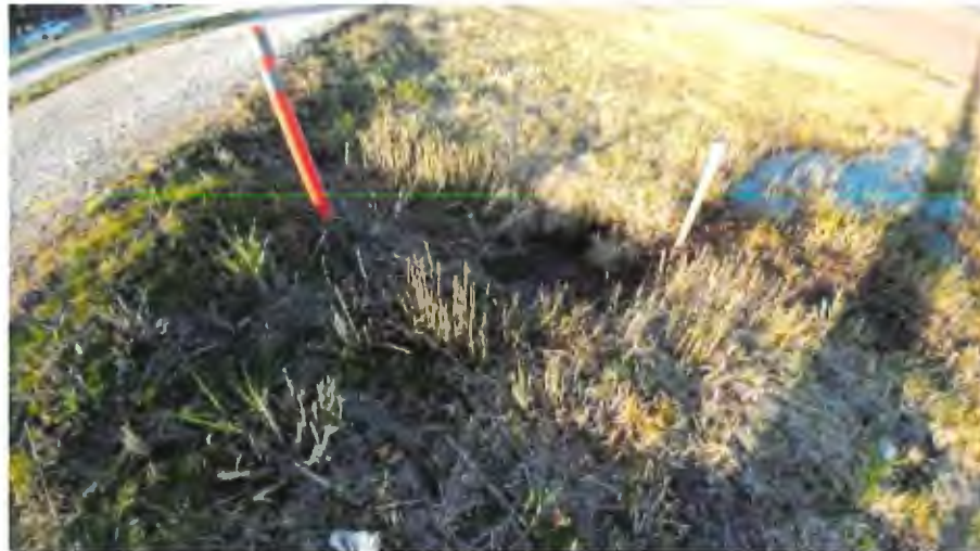
Figure 3-1: Present day not yet completed outlet the south of Lansdowne Rd. along Garden City Rd. as of March 9 th 2020.
