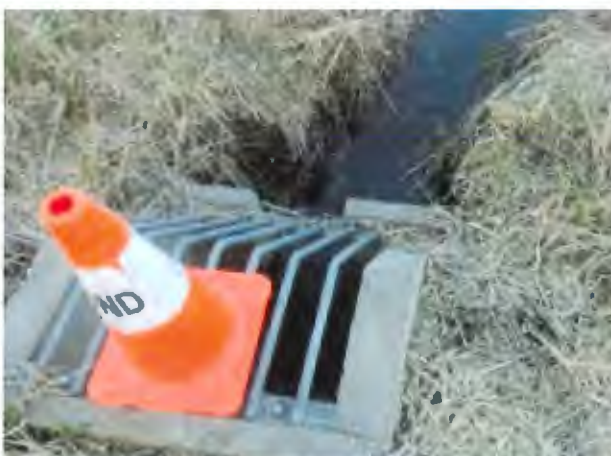
Figure 3-2: Water flowing to outlet control structure north of Lansdowne Rd as of March 9 th 2020.
