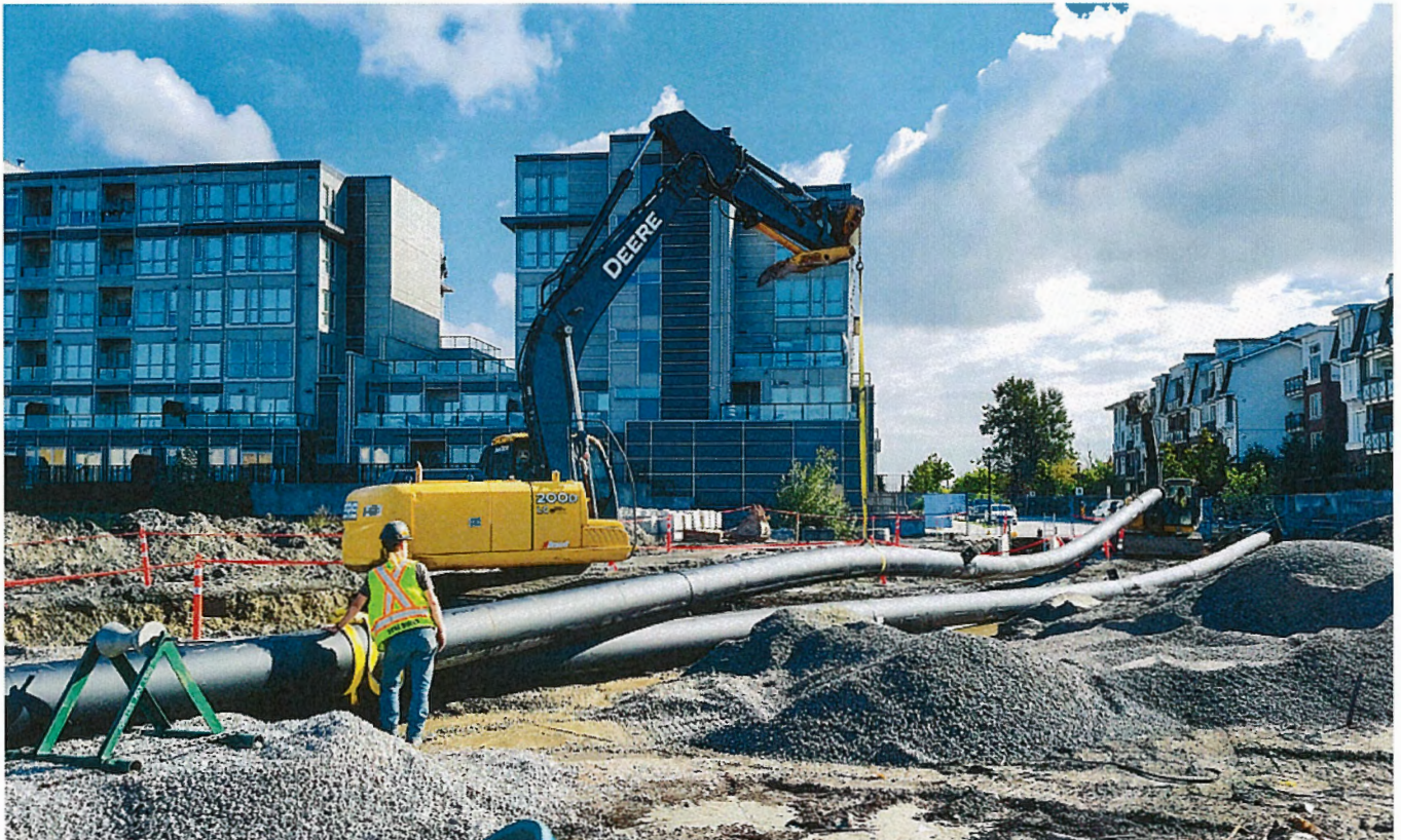
New distribution piping being installed in the Alexandra District Energy Utility service area to connect the Westmark and Berkeley House buildings
