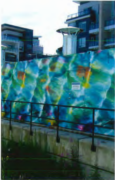
Oval Village District Energy Utility Interim Energy Centre (2020)
