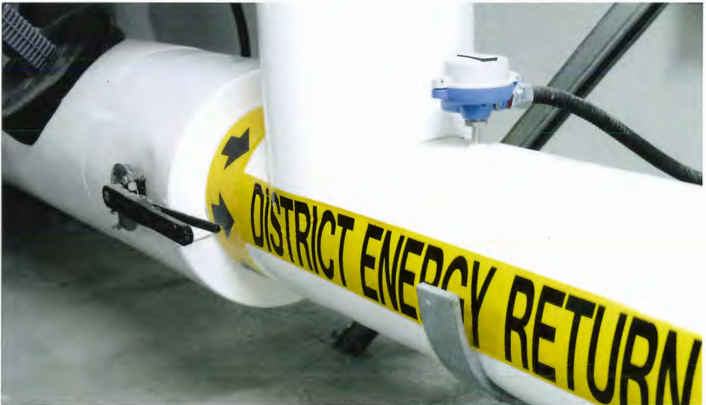
Distribution piping inside the Trafalgar building
