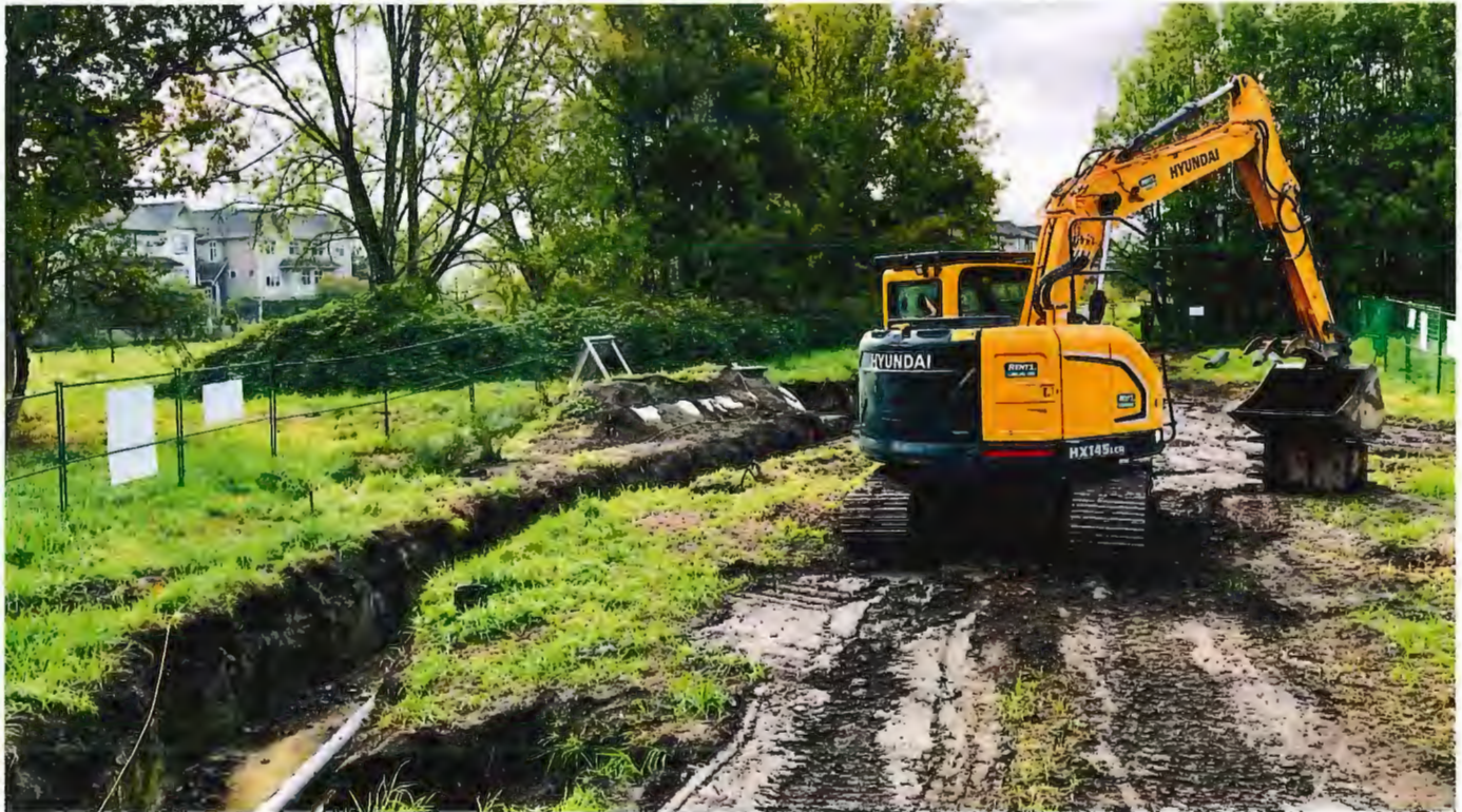
New distribution pipes being installed under Alexandra Park to allow for the future addition of new geo-exchange fields once the park is developed
