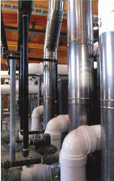
District energy infrastructure within the ADEU plant.
