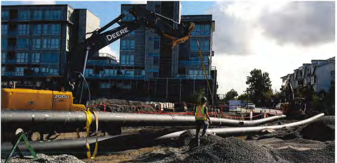
The ADEU network is further expanded to provide more customers with clean energy.
