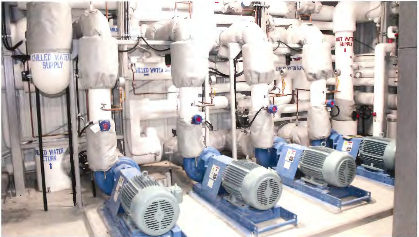
Distribution piping at the OVDEU.
