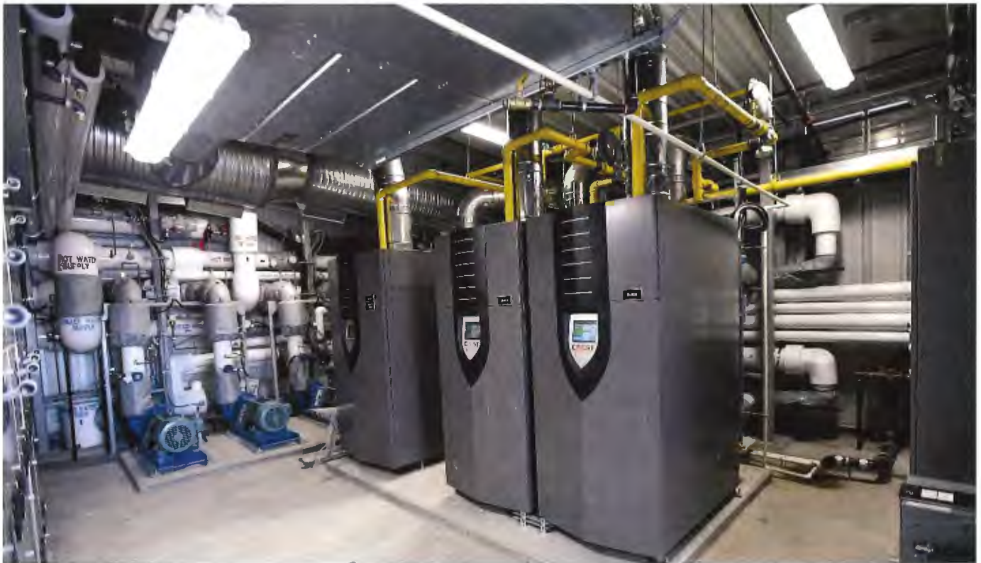
A view inside the mechanical room of a building connected to district energy services.
