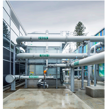
Alexandra District Energy Utility phase 4 expansion.
