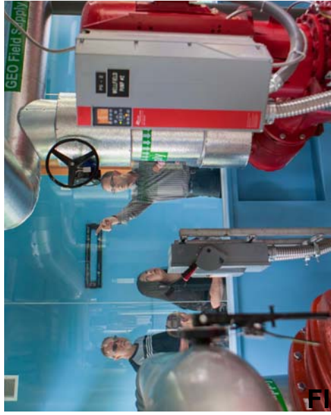
Alexandra District Energy Utility
