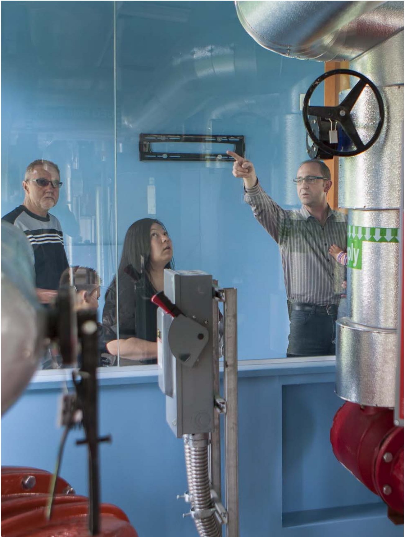
Council approved the next phase of expansion for Richmond's award-winning Alexandra District Energy Utility.
