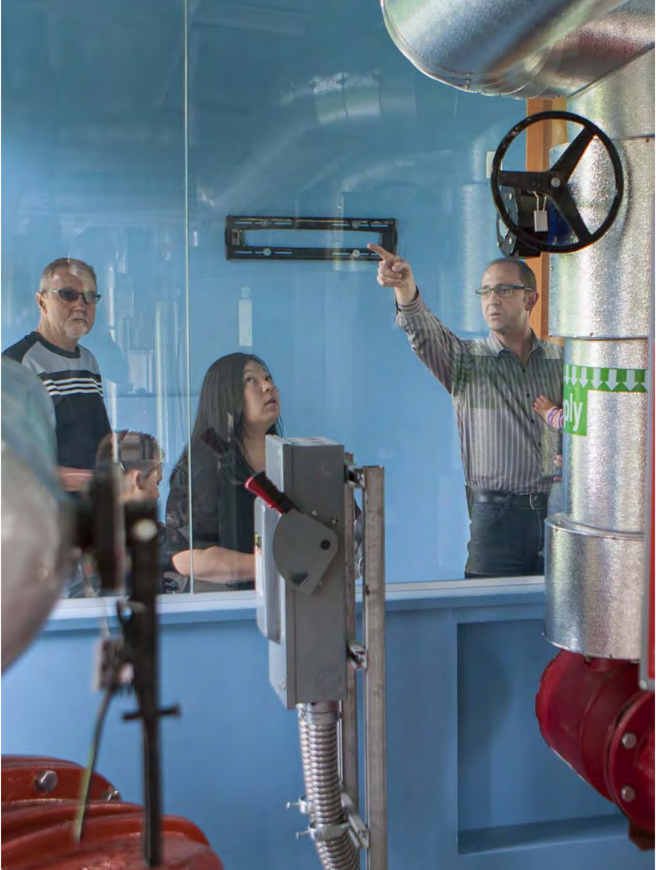
Council approved the next phase of expansion for Richmond's award-winning Alexandra District Energy Utility.
