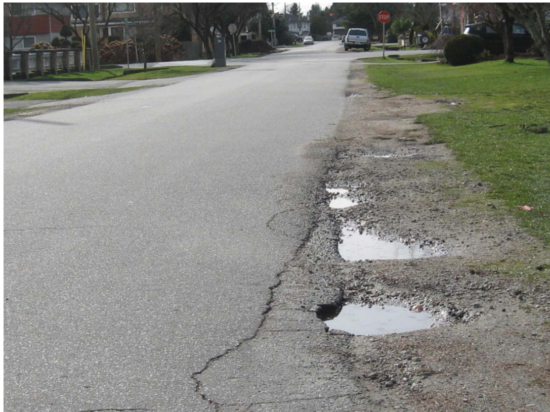
Photograph of a street where neighbourhood walkway work is required
