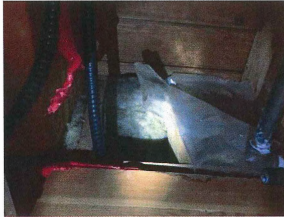
Figure 28 – Discontinuous vapour barrier.
