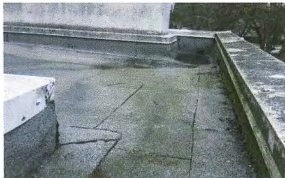
Figure 71 – Ponding water adjacent to scupper drain.
