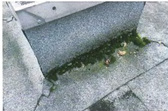
Figure 73 – Moss growth on the roofing membrane (typical).
