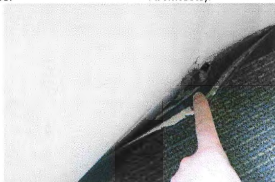
Figure 12 – Typical water ingress at the base of wall.
