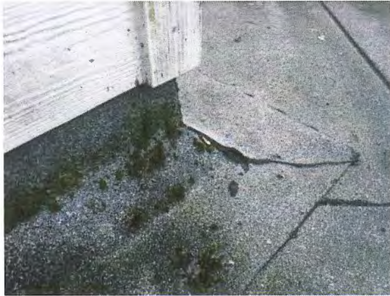
Figure 63 – Fish mouth in the roofing membrane.
