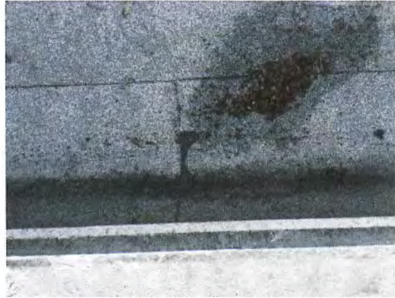
Figure 64 – Roofing membrane bleed out.
