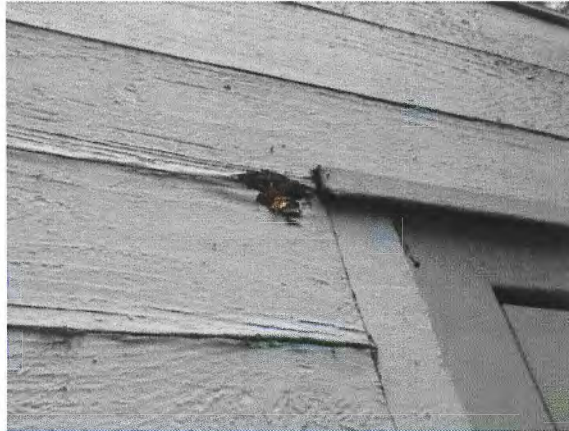
Figure 57 – Metal flashing at the door head does not incorporate an end dam. Water runoff can cause deterioration of the siding.
