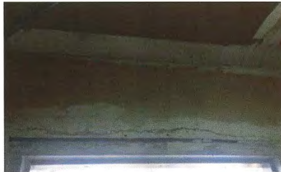
Figure 41 – Water ingress at mechanical room door head.
