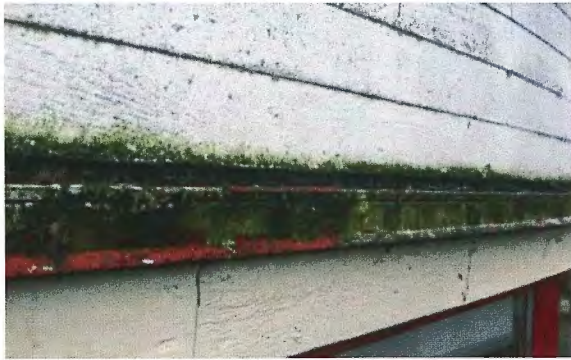
Figure 21 – Deteriorated horizontal cedar siding above window head flashing.
