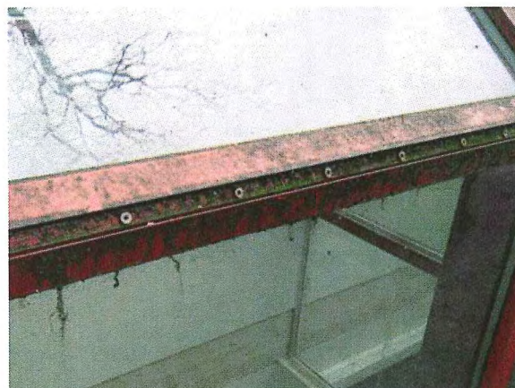
Figure 50 – Corroding fasteners at skylight (typical).
