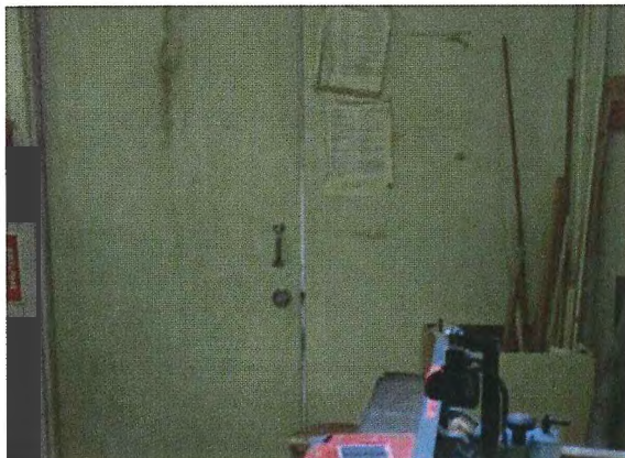
Figure 46 – No gasket around the door and daylight is visible through the door slabs.
