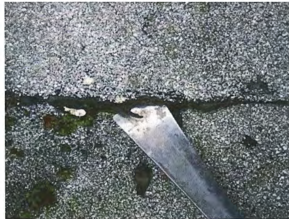
Figure 66 – Failed roofing membrane seams.
