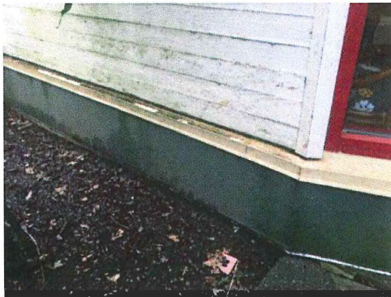
Figure 10 – Typical base of wall finished grade near the top of the slab on grade.
