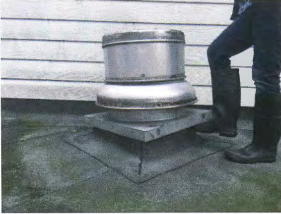
Figure 77 – Extraction fan not well secured
