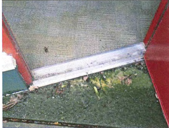
Figure 44 – Corroding fasteners at door threshold (typical).
