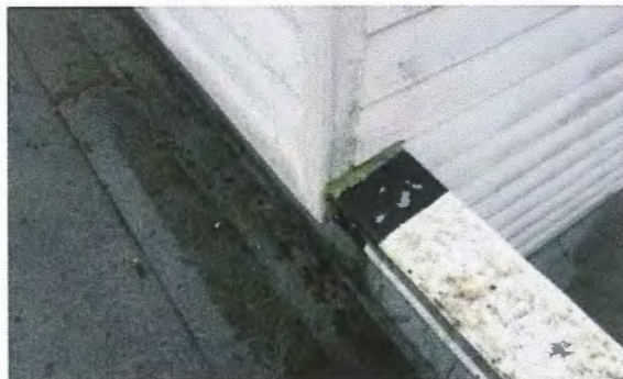
Figure 76 – Suspect saddle interface and exposed self-adhered membrane.
