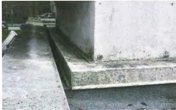
Figure 79 – Roof vent in close proximity to the roof parapet.
