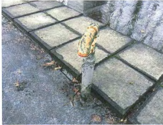
Figure 81 – Roof access vent relies on single sealant.
