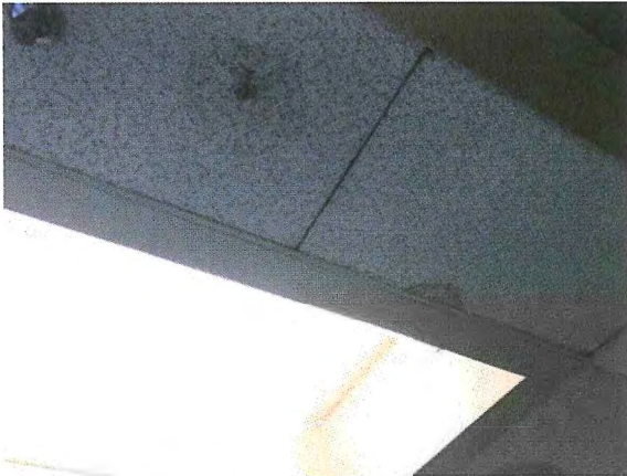
Figure 51 – Signs of water ingress at skylight.
