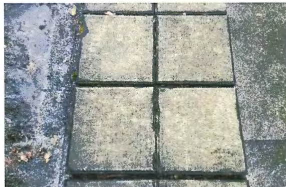
Figure 72 –Debris between roof pavers and obstructed drainage.
