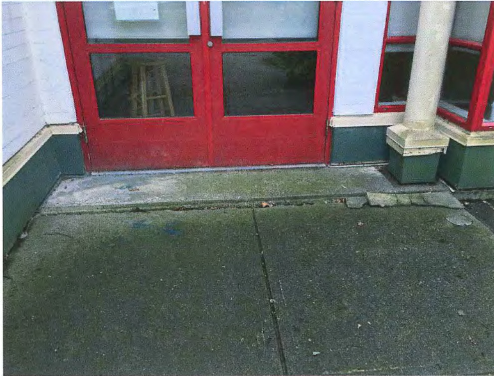
Picture 5 - Ground settlement at several door thresholds. Edge of raft slab exposed creating a cold bridge.
