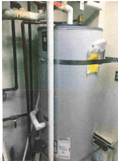
Figure 5 – Existing indirect DHW heater/tank
