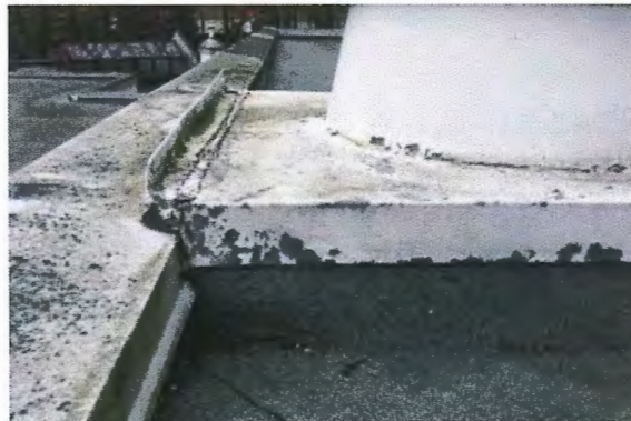
Figure 75 – Delaminating paint at metal flashing.
