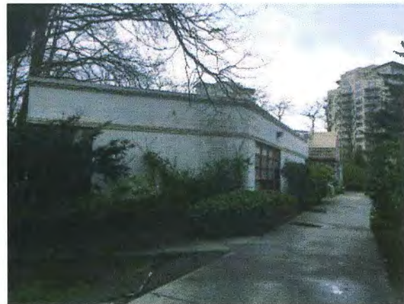
Figure 27 – Vegetation in close proximity to the exterior walls.
