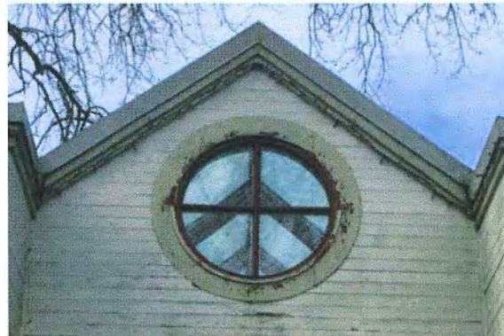
Figure 18 – Delaminating paint finish on the horizontal cedar siding.
