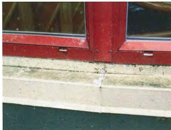
Figure 56 – Metal flashing seam unsealed and only overlapped.
