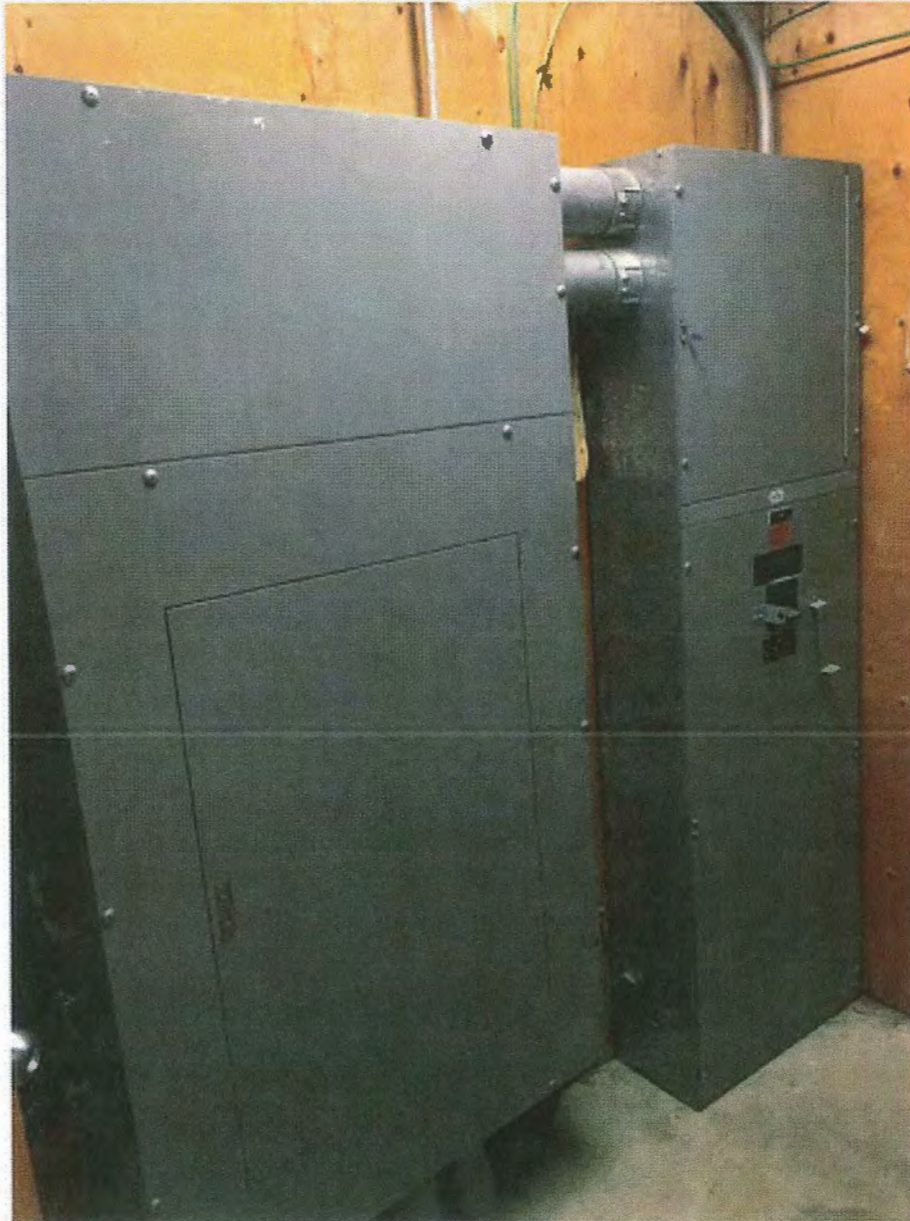
Figure 2 – Building Main Switchboard 800A
