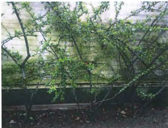
Figure 26 – Vegetation in close proximity to the exterior wall and staining on the cladding.
