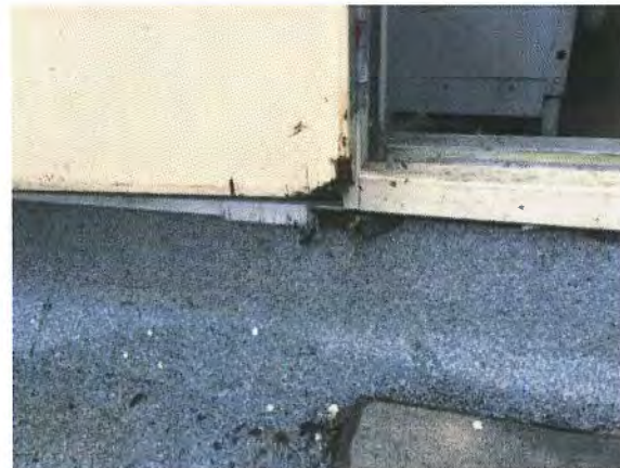
Figure 68 – The roofing membrane not extending into door rough opening and has exposed edge.
