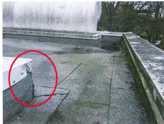
Figure 67 – Metal flashing cutting into the roofing membrane.
