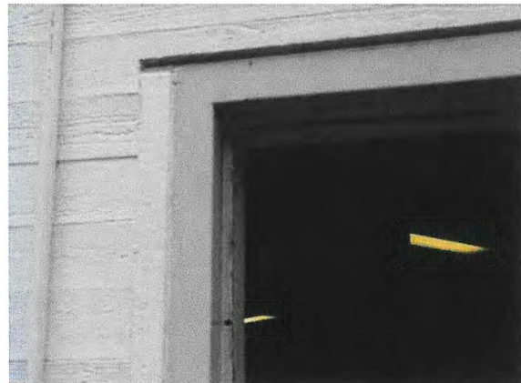
Figure 47 – No gasket around the door.
