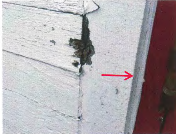
Figure 35 – Failed sealant around window.
