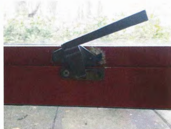
Figure 32 – Broken window hardware.
