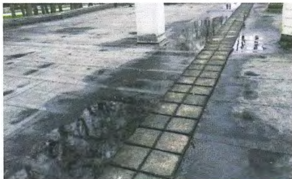
Figure 70 – Ponding water within the field of roof where pavers are obstructing drainage.
