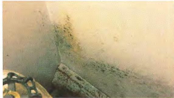
Figure 14 – Signs of water ingress in the sprinkler room, below the glass canopy to wall interface on the north-east elevation.
