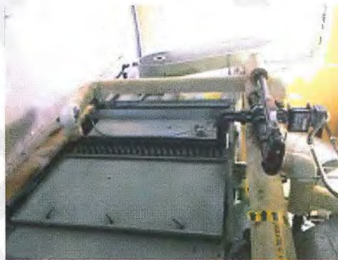
Figure 2 – Existing indoor AHU
