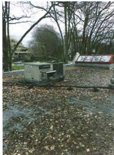
Figure 4 – Existing rooftop unit
