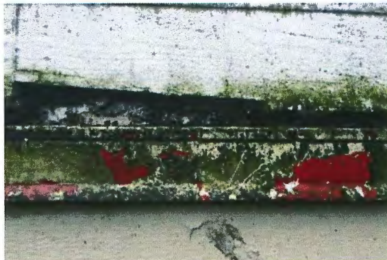
Figure 17 – Delaminating paint on metal flashing.
