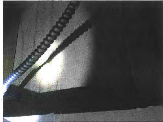
Figure 52 – Signs of water ingress at skylight.
