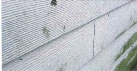
Figure 24 – Failed sealant at joint in the cementitious horizontal siding.
