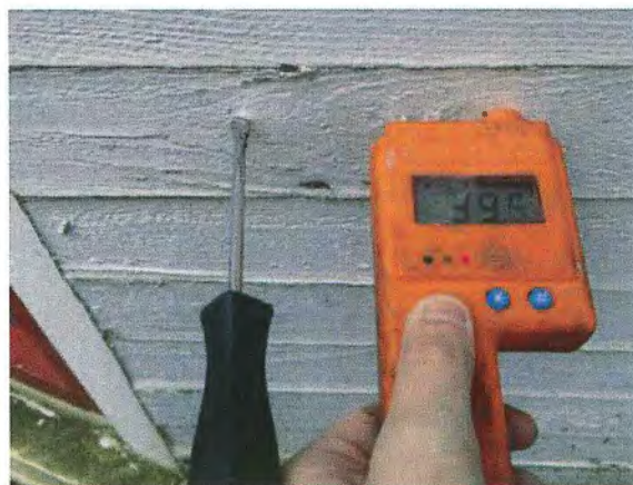
Figure 23 – Elevated moisture content and deterioration of horizontal cedar siding.
