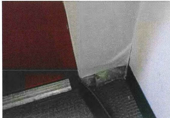
Figure 45 – Water ingress at door sill.
