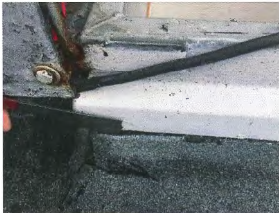
Figure 69 – Exposed edge of roofing membrane.
