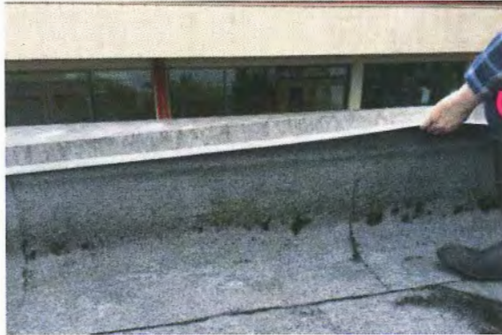
Figure 74 – Roof parapet metal flashing not well-secured.
