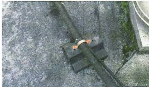
Figure 82 – Corroded fasteners at electrical cables.
