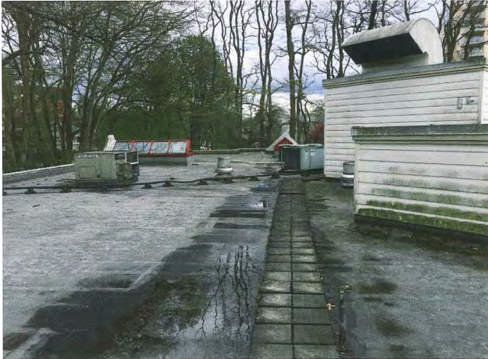
Picture 3 - Roof in Fair Condition – Drains Well. There are several Rooftop Units.
