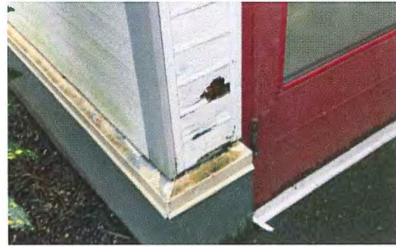
Figure 22 – Deteriorated horizontal cedar siding.
