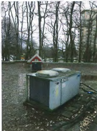
Figure 3 – Existing outdoor Split Condensing
