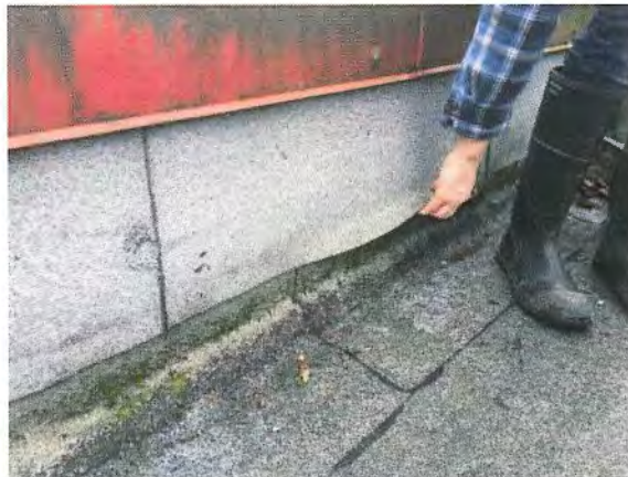
Figure 65 – Roofing membrane not well adhered.
