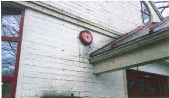
Figure 13 – Suspect detailing at the glass canopy to wall interface next to the main entrance on the north-east elevation.
