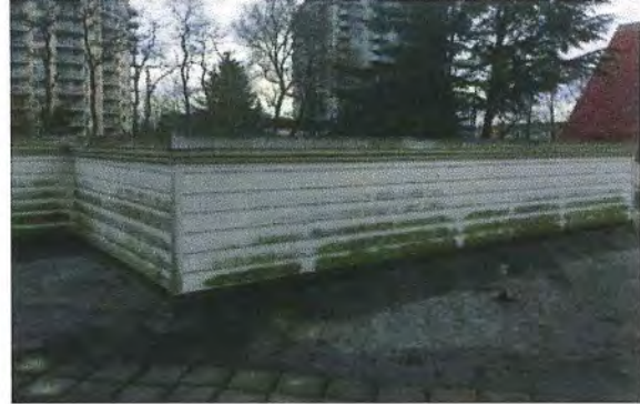
Figure 20 – Stained cementitious horizontal siding at the roof.
