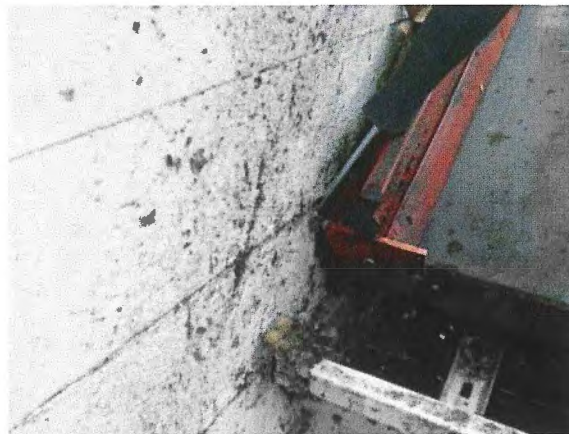
Figure 53 – Poor detailing at glass canopy to wall interface and deterioration of horizontal cedar siding.
