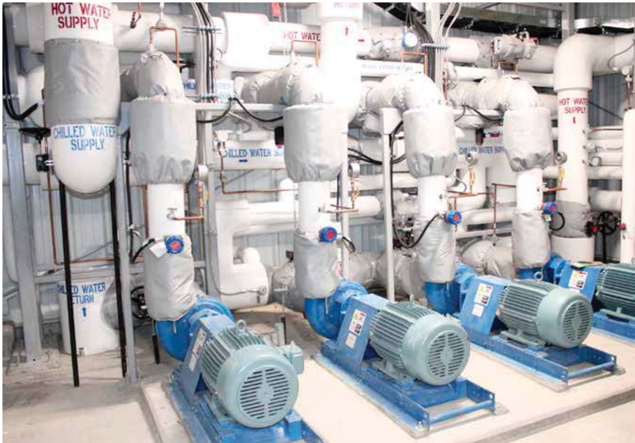
The Alexandra District Energy Utility was expanded to provide service to a major new retail complex.
