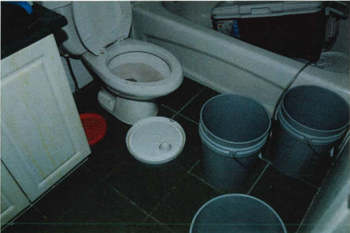
Image 5: chemicals in upstairs bathroom, chemical staining on cabinets and colour of toilet water suggest dumping of waste into sewer system
