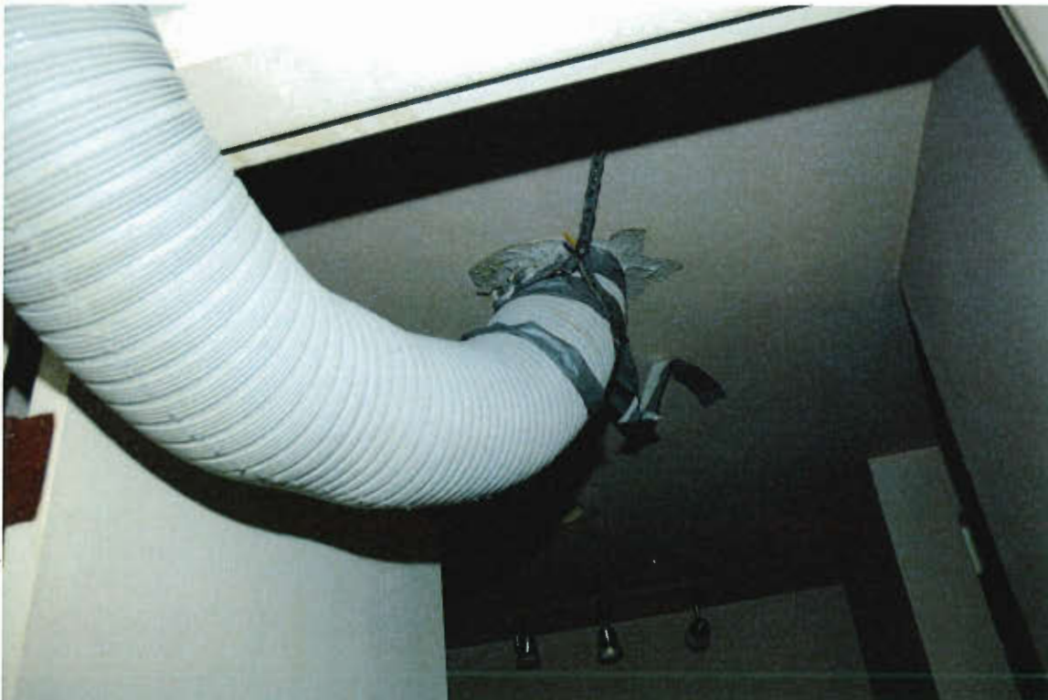
Image 7: tubes used as venting of chemical vapours into attic
