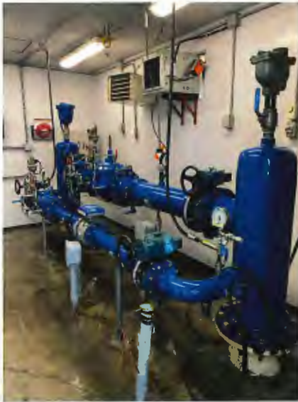
Nelson Road PRV Station
