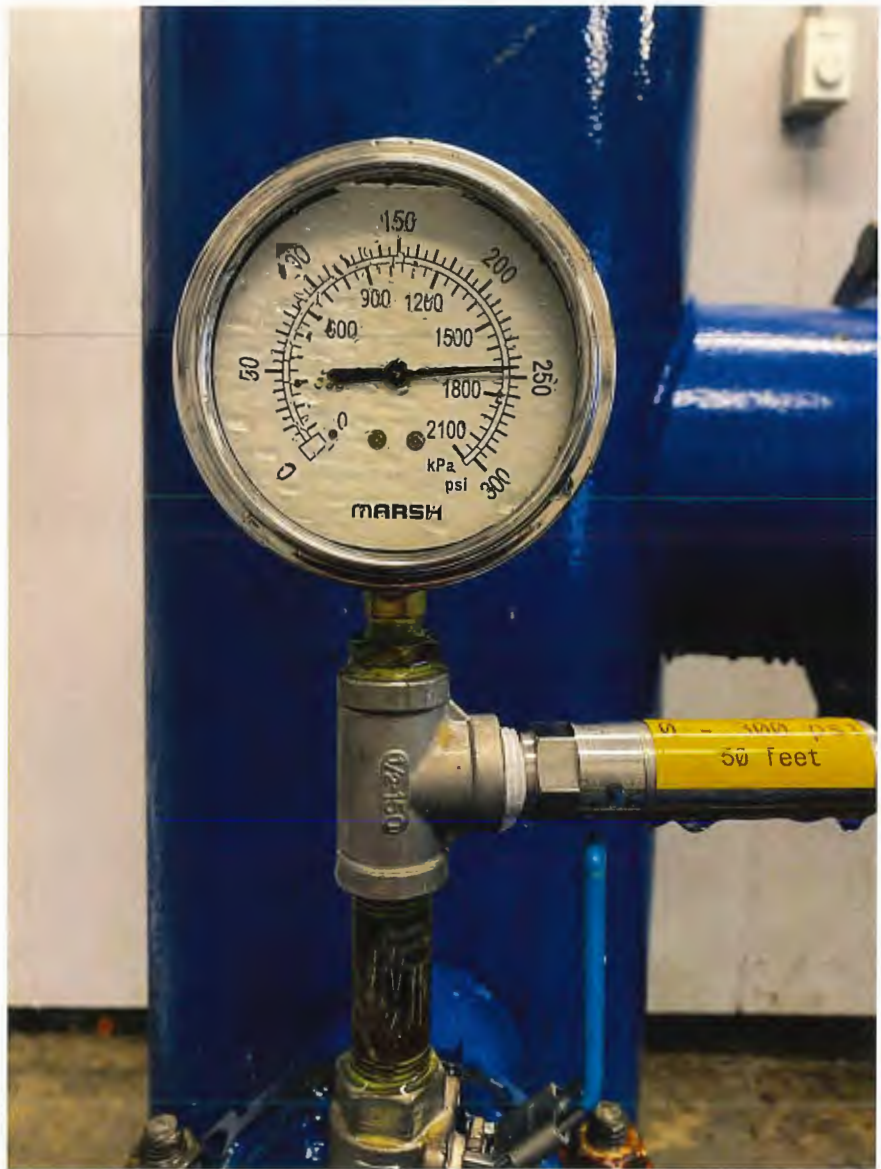
Metro Vancouver water connection to PRV station
