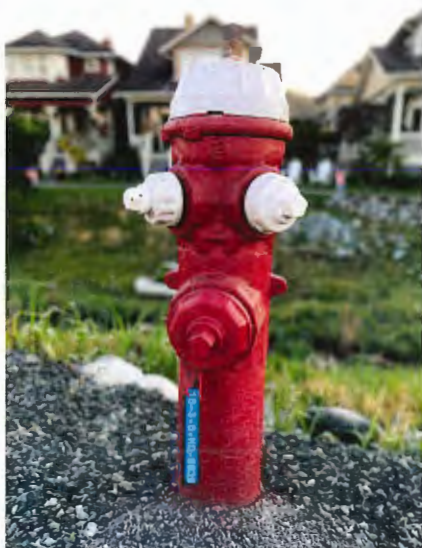
Tagged fire hydrant
