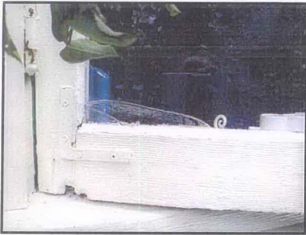
Windows: Broken pane
