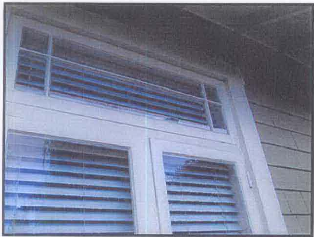
Windows: Broken top pane
