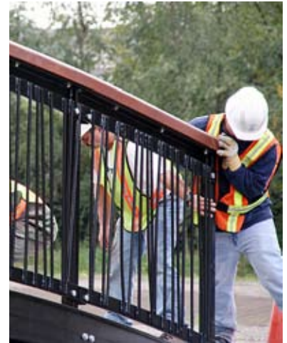
A foot bridge was installed over the pond at the new Garden City Community Park.
