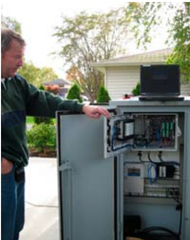
Innovative wireless technology monitors Richmond's critical drainage system around the clock.
