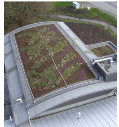
Green roofs are one of many sustainability features of Richmond's new Sea Island and Hamilton Fire Halls, which officially opened in 2007.
