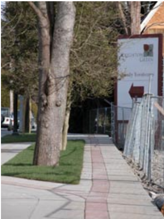
New sidewalk treatment on Garden City, looking north from General Currie Road
