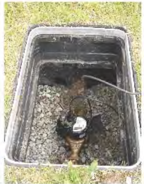
Single-family water meter
